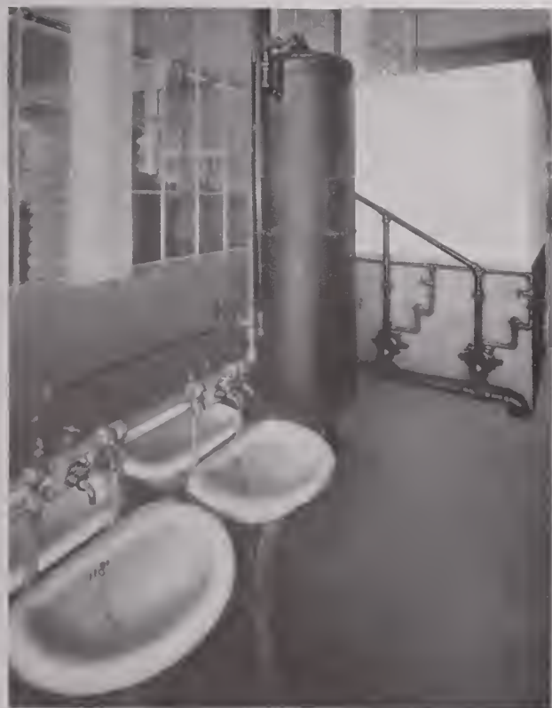
HOT WATER FOR LAVATORIES
